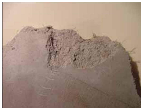
Broken asbestos insulation board containing amosite.
